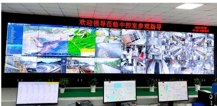
Fig. 1: Chengyu Digital Mine system central control room
